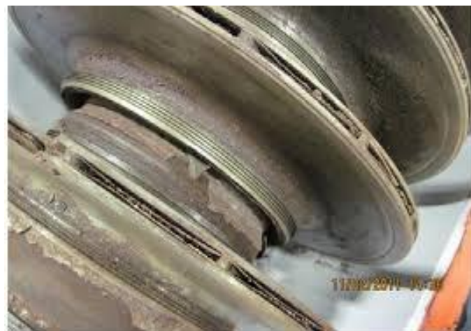
Image 1.2 Fouling and corrosion
