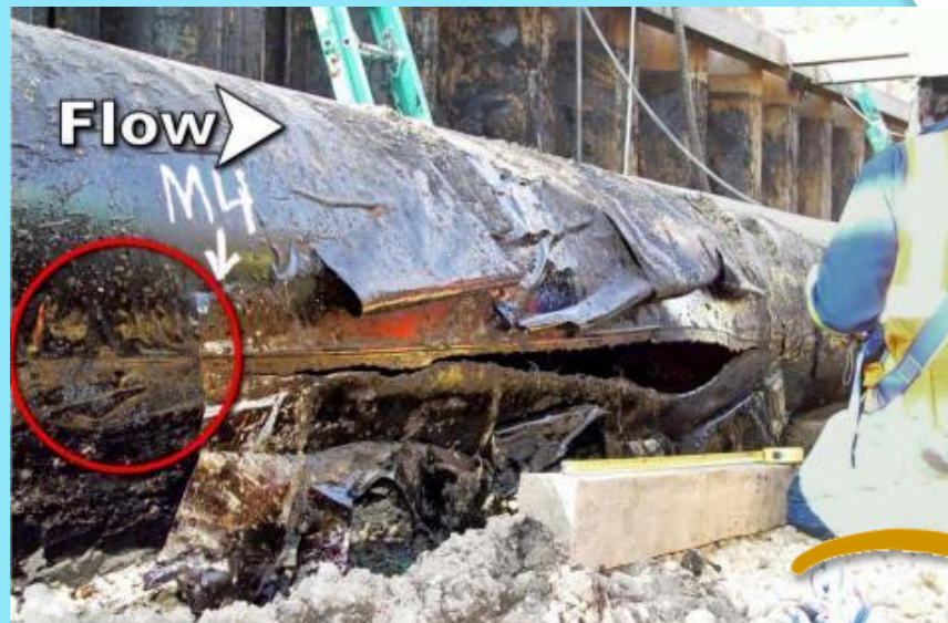
30 INCH PIPE RUPTURE (ENBRIDGE ENERGY)
